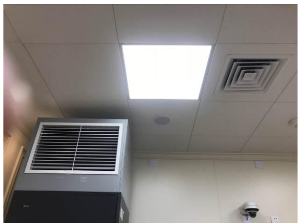
(机房顶部新风口)
